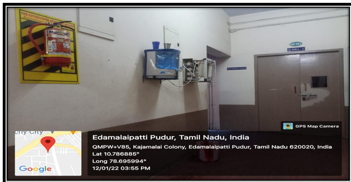
REVERSE OSMOSIS (RO) WATER & FIRE EXTINGUISHER FACILITIES
